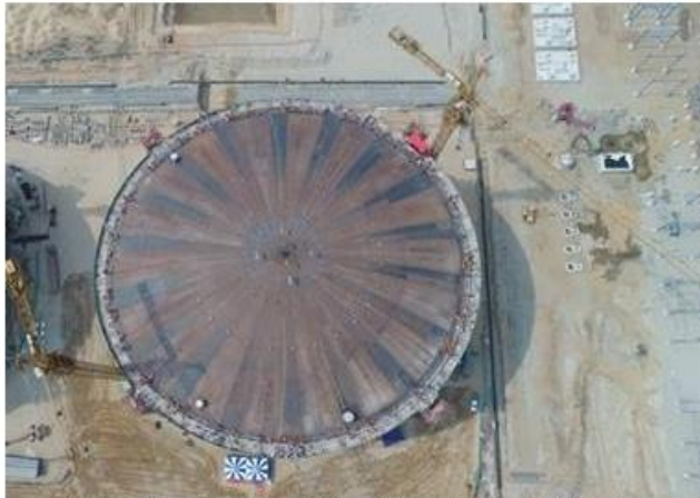
Final position of tank roof after raising at a height of 40 mtrs.
